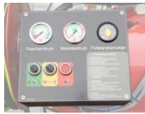
Control panel with electrical filling level indication
