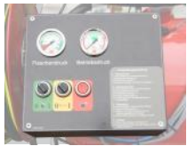
Control panel without electrical filling level indication
